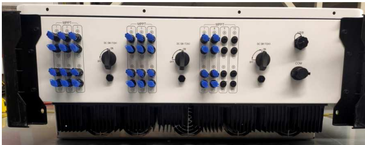
PV Input Terminal view
